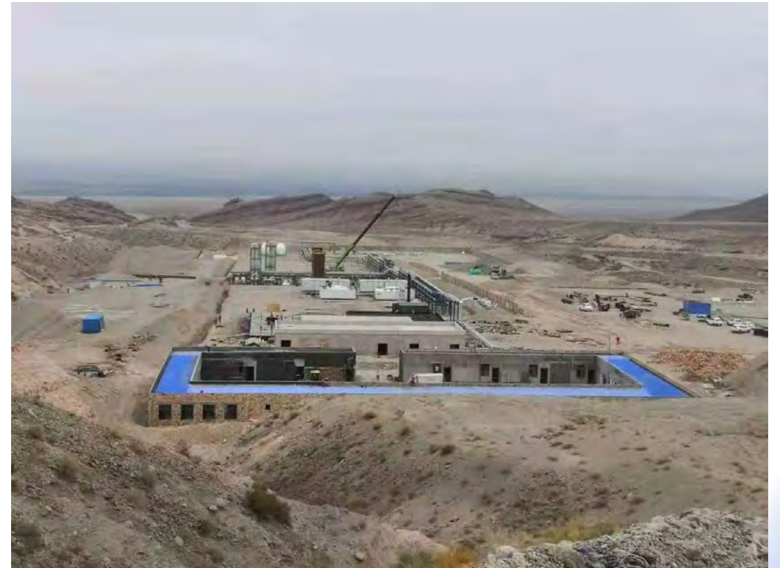
Tudong Well No. 2, Phase I, 2 \times 6 \times 10^4 \text{Nm}^3/\text{d} LNG plant, Design and Photo
